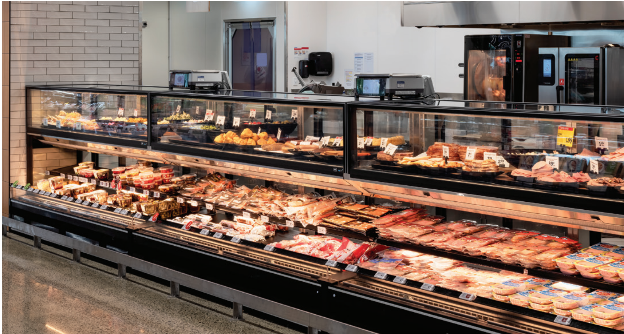
NEW WORLD HOBSONVILLE, NEW ZEALAND - ISOFORM GRAB&GO REFRIGERATED/REFRIGERATED 2400 (MULTIPLXED)
