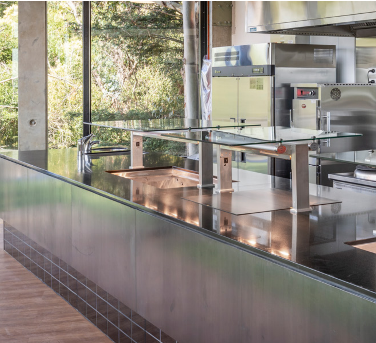
WAIPARURU HALL AUCKLAND UNIVERSITY - INLINE GN SERIES IN-COUNTERS UNDER-MOUNT WITH FLAT SELF-SERVE GLASS GANTRY
